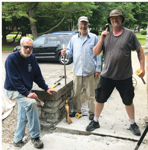
Steve Hilsdorf and crew repairing the sidewalk by the side entrance to FBC. Photo from Debbie Bennett Reynolds
