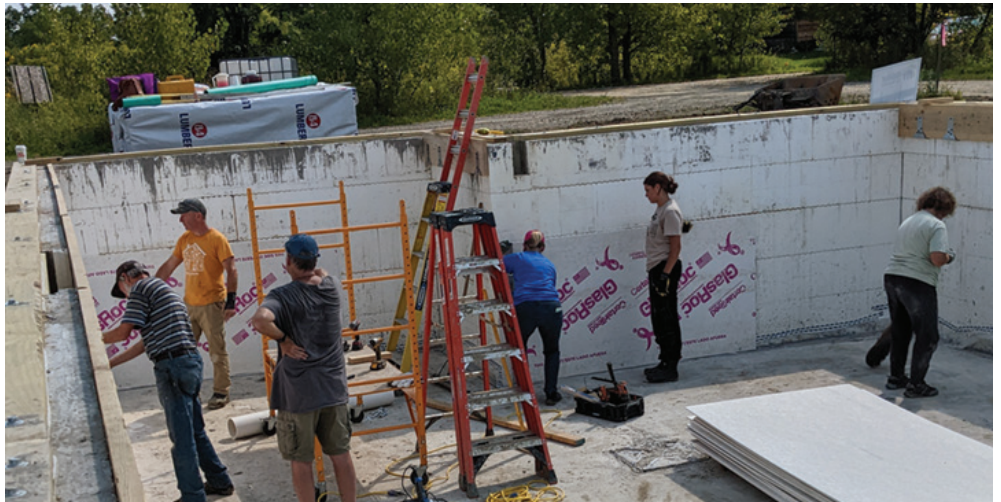
FBC adult volunteers work on wall boarding a basement of a new Habit of Humanity home.
